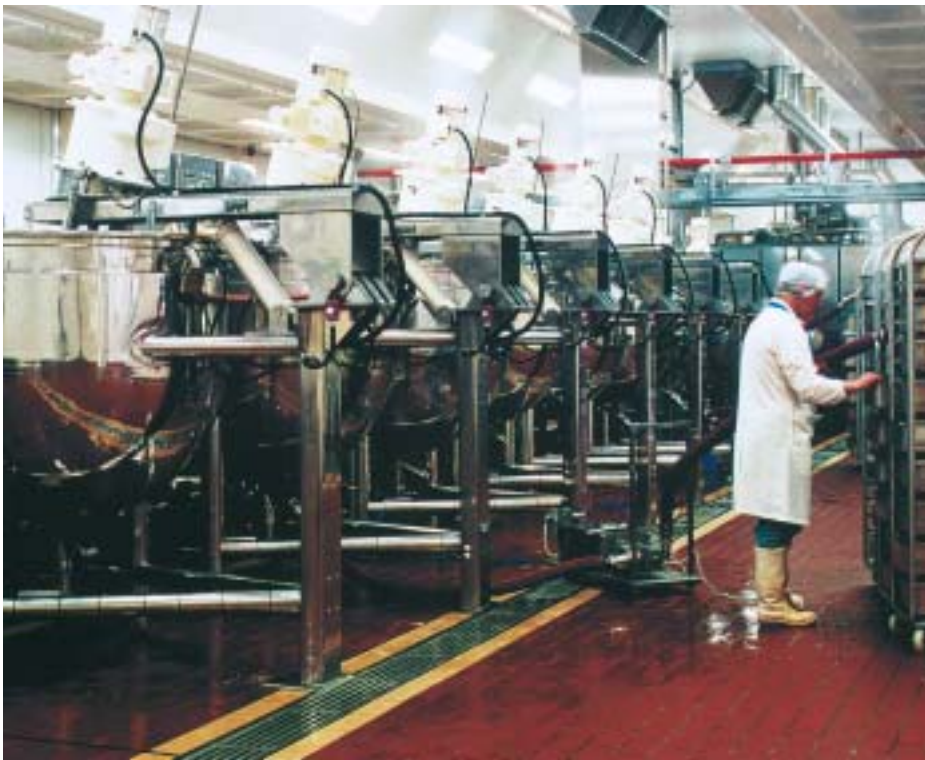
Sauce processing: Hy-Mix kettle installation similar to the new plant commissioned at Fisher Foods
