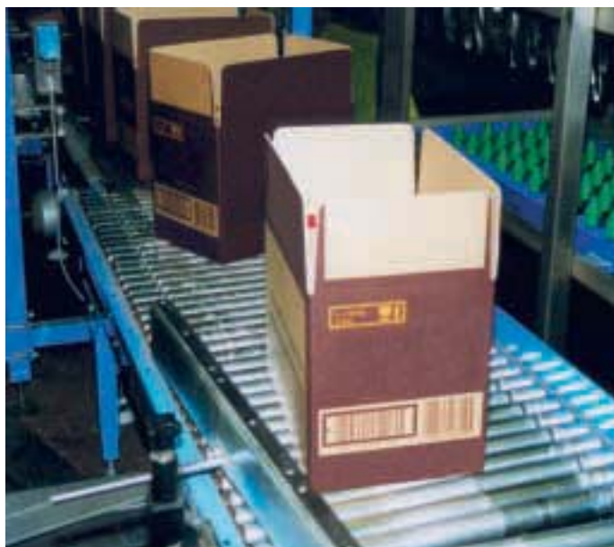
Case delivery: Part of the CSL system installed at a major distillery
