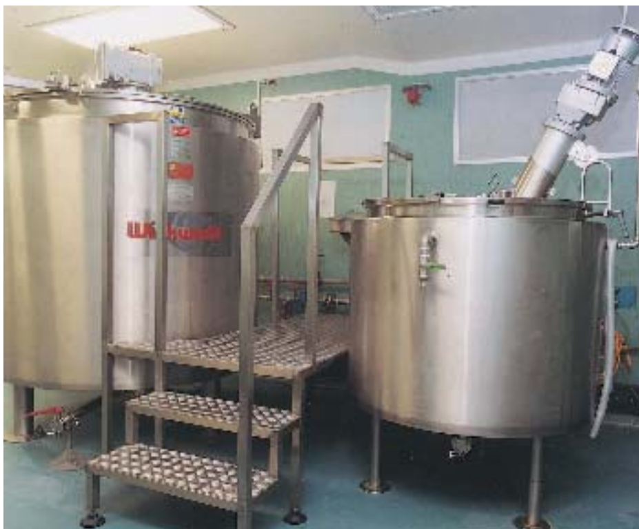
Extra flexibility: Pharmasol has installed two custom mixing vessels, purpose built by Winkworth Machinery
