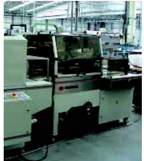
Variety of work: Rochman automatic L-sealer installed at Jet UK by Yorkshire Packaging
