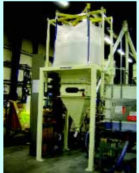
Unloading sand: Spiroflow bulk bag discharger and conveyor system at Carroll & Meynell
