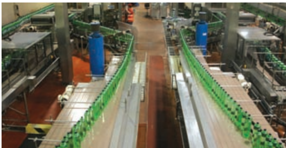
At Wakefield, monitoring and targeting water and energy are key themes at the site
