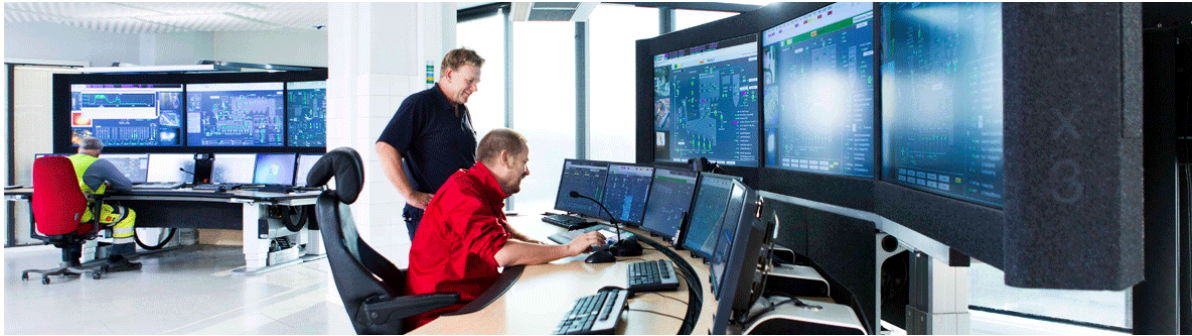
Figure 6: The modern control room. Image credit ABB
